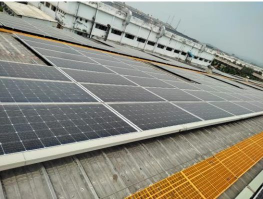
1000 KWP Roof Top Solar Plant
