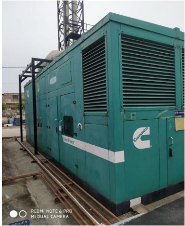
5520 kVA Capacity DG Sets (Backup Power Source)
